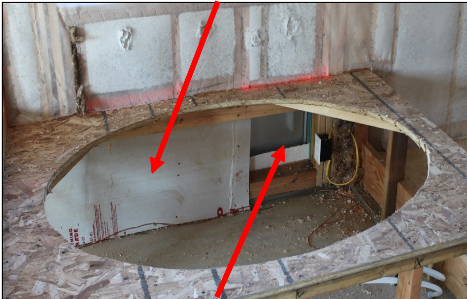
Metal access door needs to be insulated.
