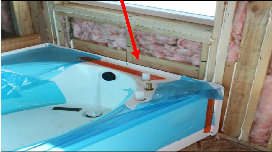
No air barrier behind tub.
